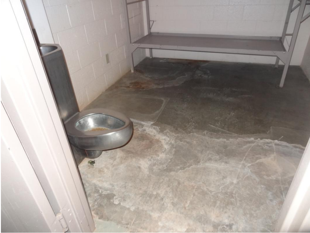
Housing Unit 7 - Building #0187 Description: Water damage from plumbing leaks.
