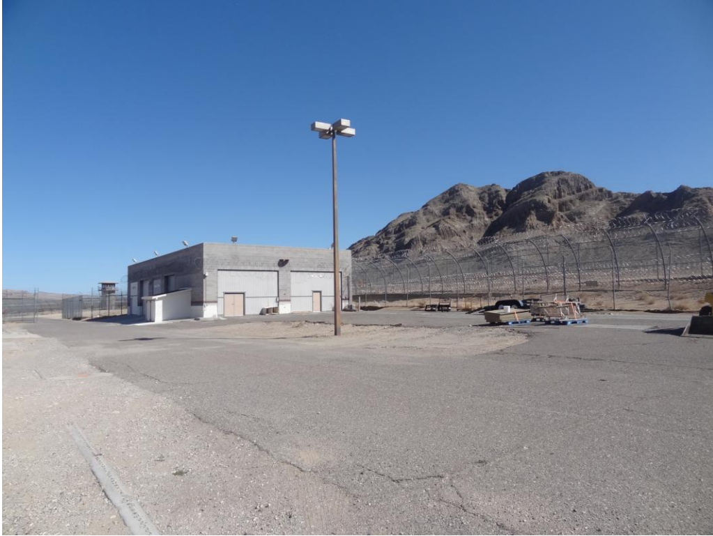
Southern Nevada Correctional Center Site - Site #9994 Description: AC paving in need of replacement.
