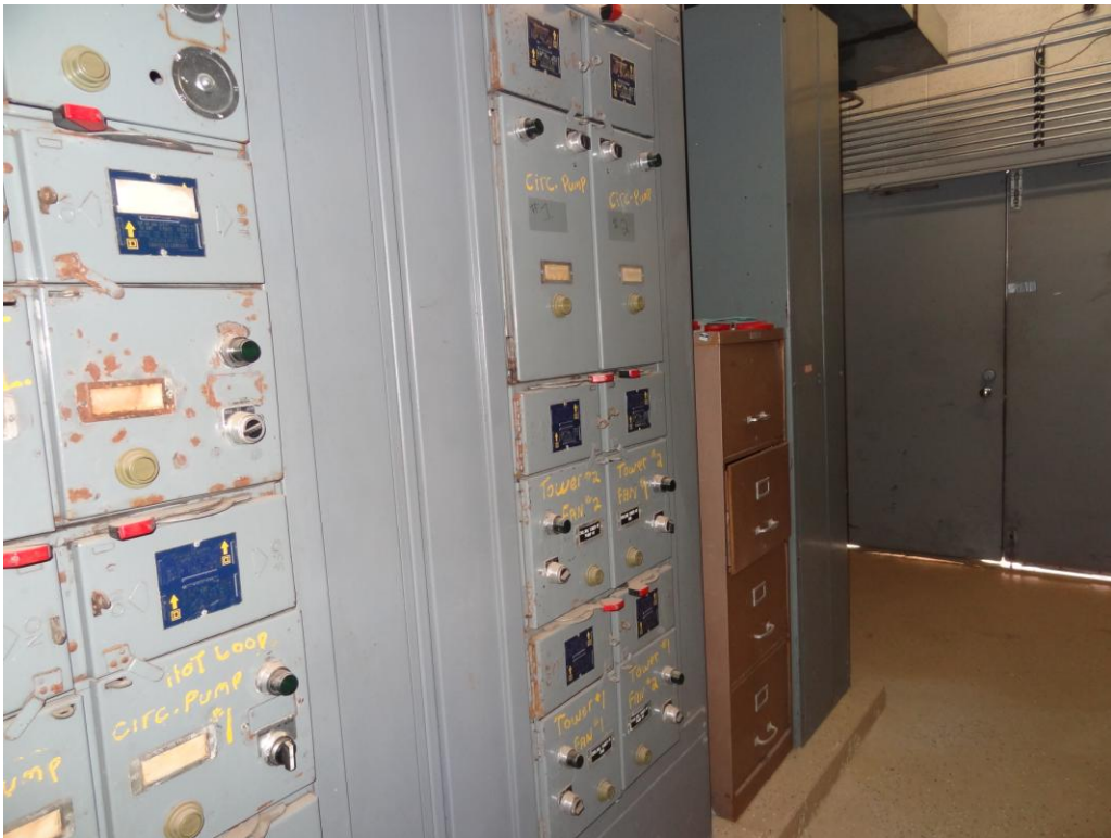
Culinary/ Dining/ Central Plant - Building #0190 Description: Electrical equipment in need of replacement.
