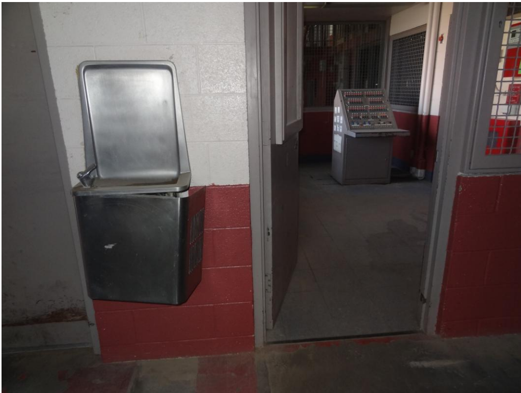
Housing Unit 5 - Building #0184 Description: Broken drinking fountain.
