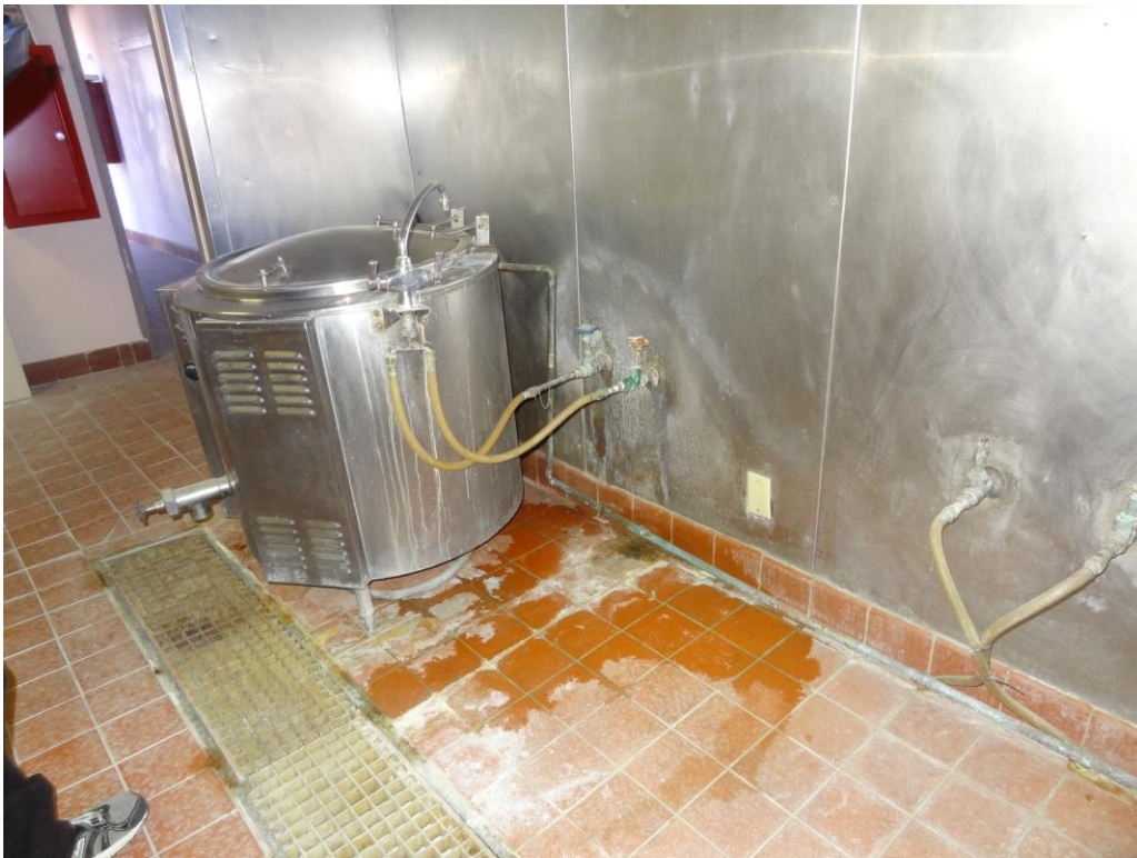
Culinary/ Dining/ Central Plant - Building #0190 Description: Damaged and missing cooking equipment.
