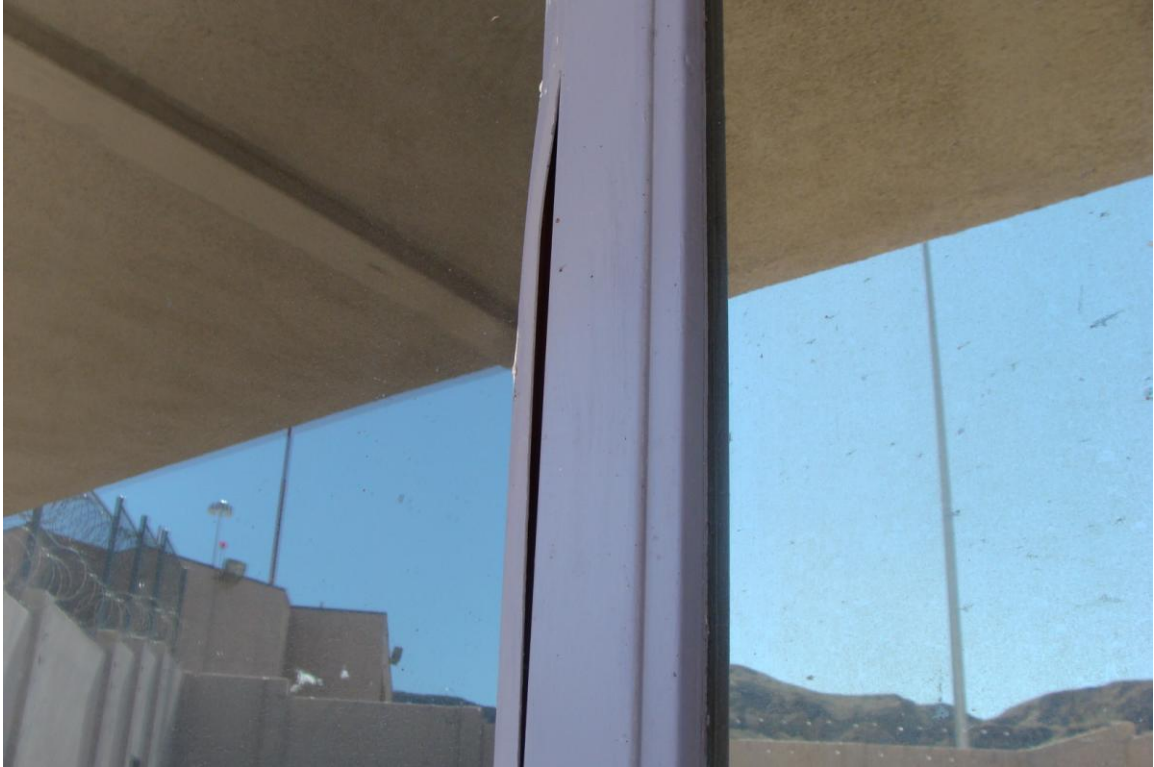
Administration / Visitation - Building #0176 Description: Damaged curtain window glazing stops.
