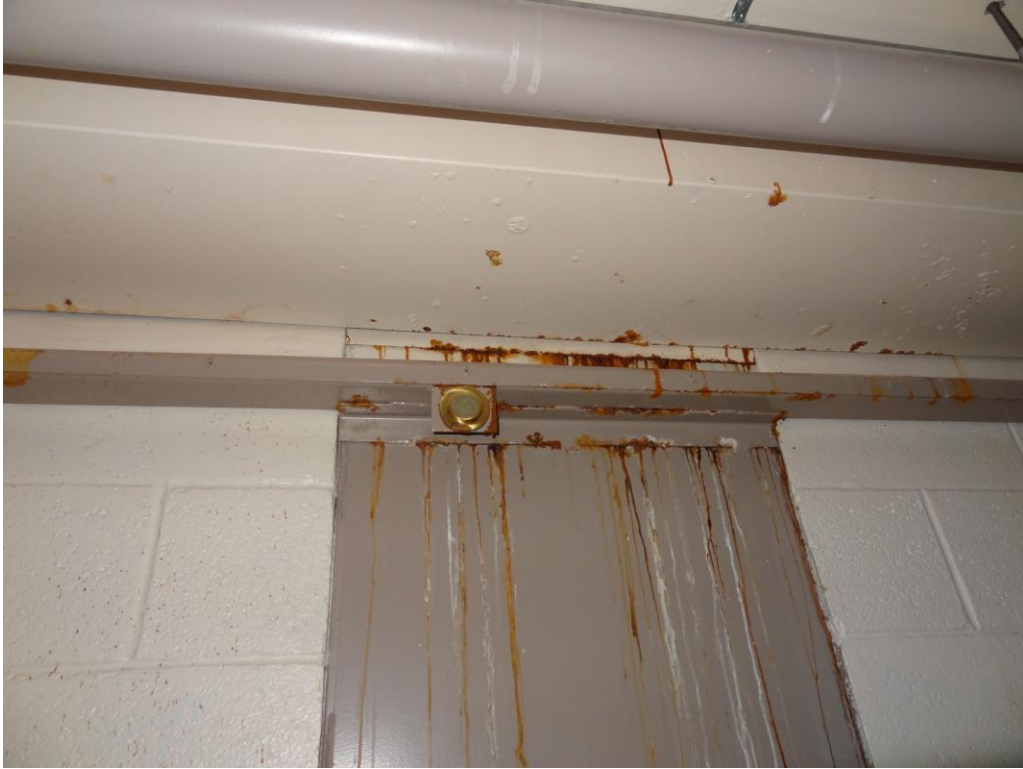
Housing Unit 5 - Building #0184 Description: Water damage from leaking pipes.
