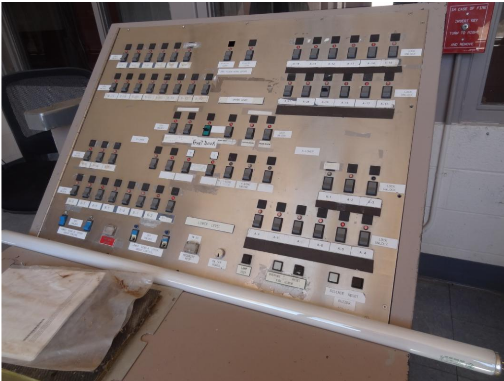
Housing Unit 7 - Building #0187 Description: Control panel in need of upgrade.
