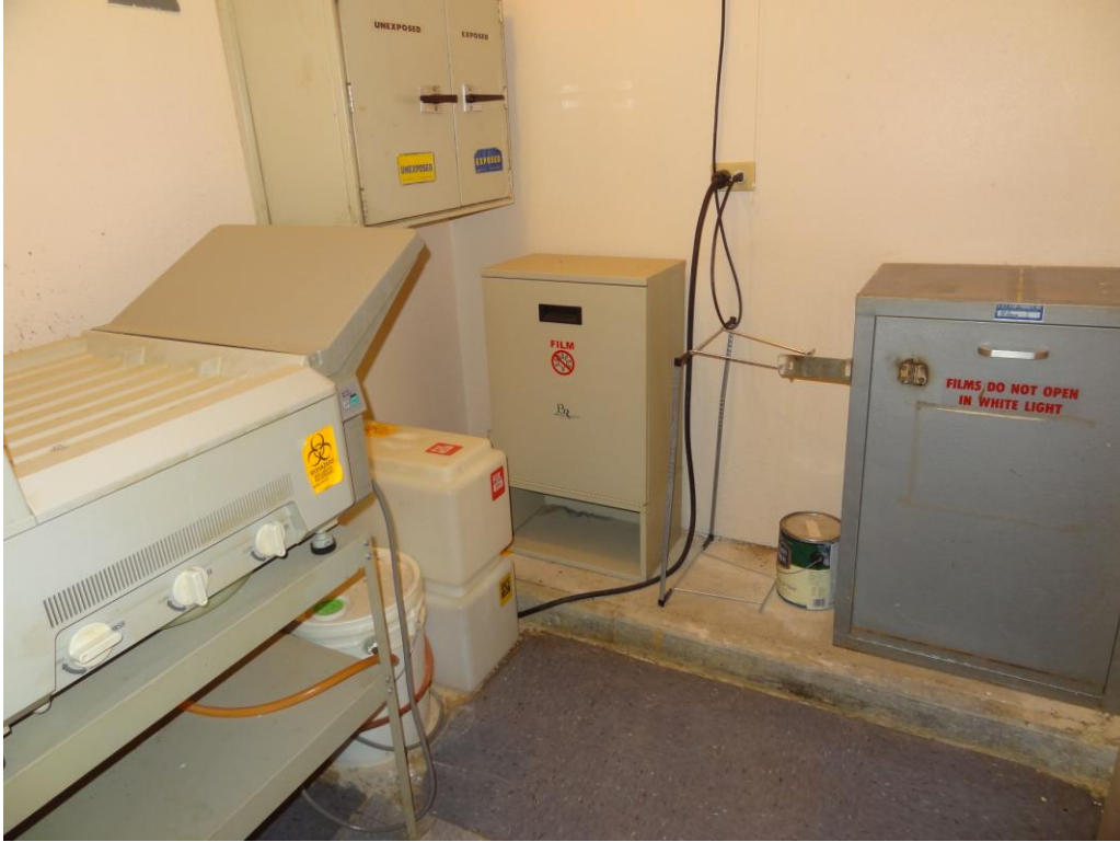
Medical Unit 8 - Building #0188 Description: Outdated medical equipment.
