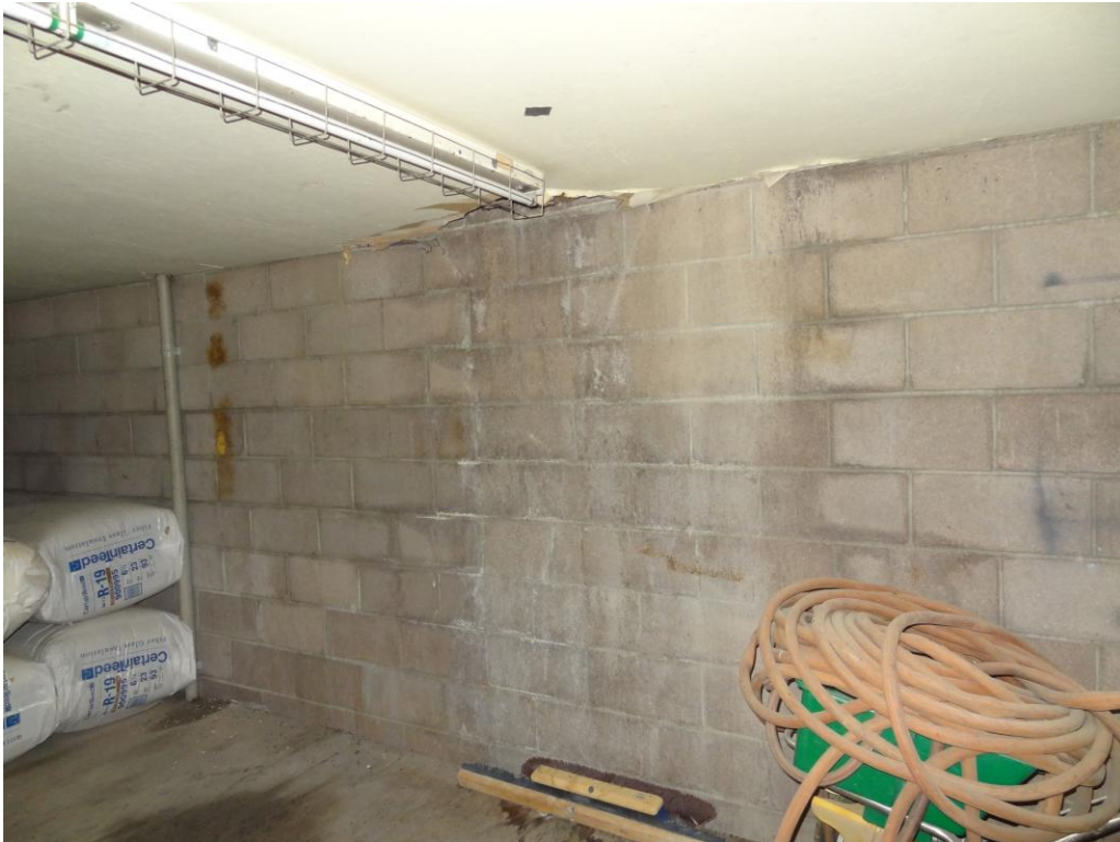
Auto Maintenance Shop/ Warehouse - Building #0192 Description: Interior of the building with water damage.
