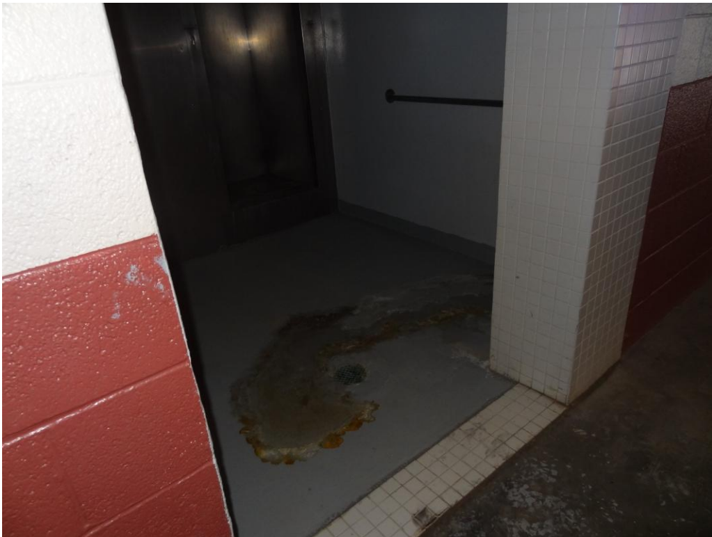
Housing Unit 6 - Building #0185 Description: Water damage in shower area.
