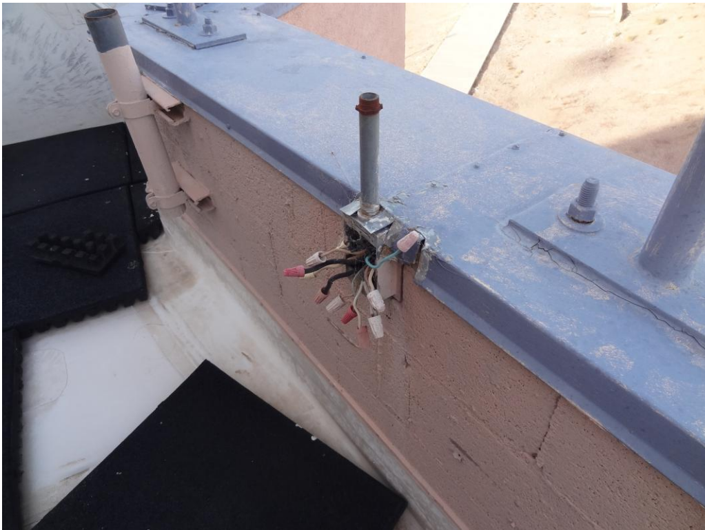
Recreation/ Gym - Building #0186 Description: Roof mounted electrical box in need of cover plate.
