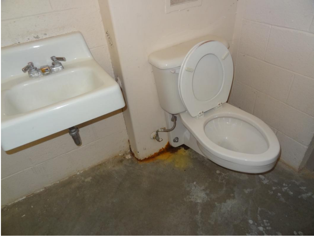
Housing Unit 1 - Building #0180 Description: Water damage from leaking pipes at cell fixtures.
