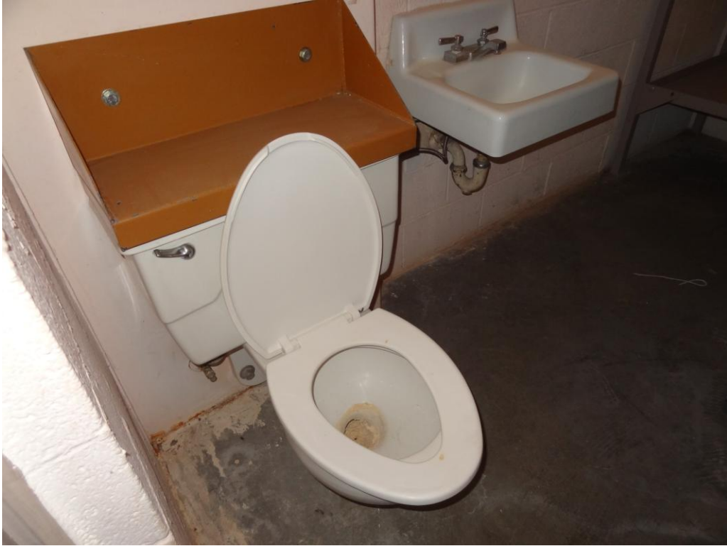
Housing Unit 3 - Building #0182 Description: Porcelain fixture in cell with dried out water closet.
