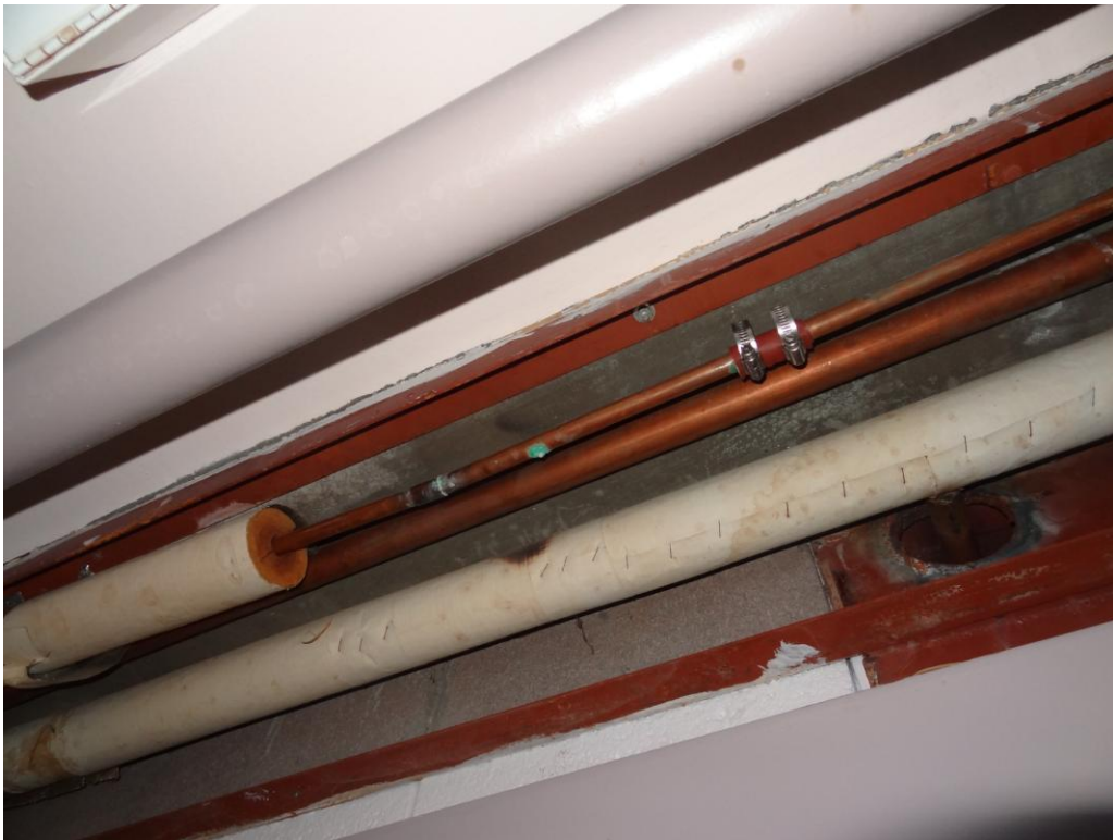
Housing Unit 3 - Building #0182 Description: Active and repaired pinhole leaks in copper plumbing.
