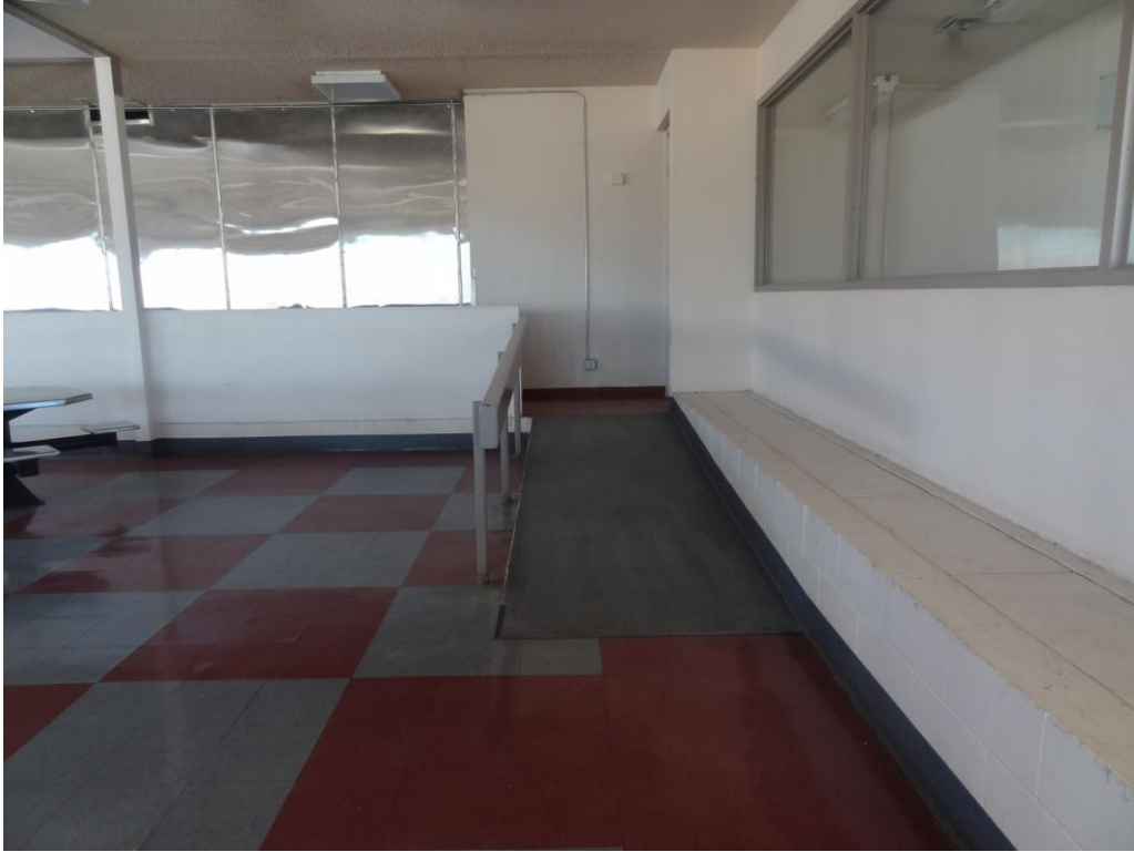
Culinary/ Dining/ Central Plant - Building #0190 Description: Non-ADA compliant ramp in dining.
