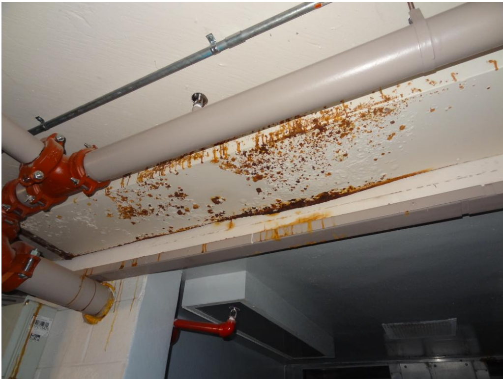
Housing Unit 1 - Building #0180 Description: Water damage from leaking pipes.
