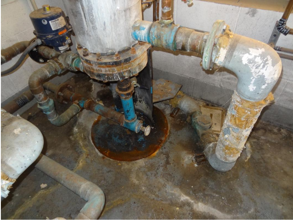
Culinary/ Dining/ Central Plant - Building #0190 Description: Central Plant equipment in need of replacement.
