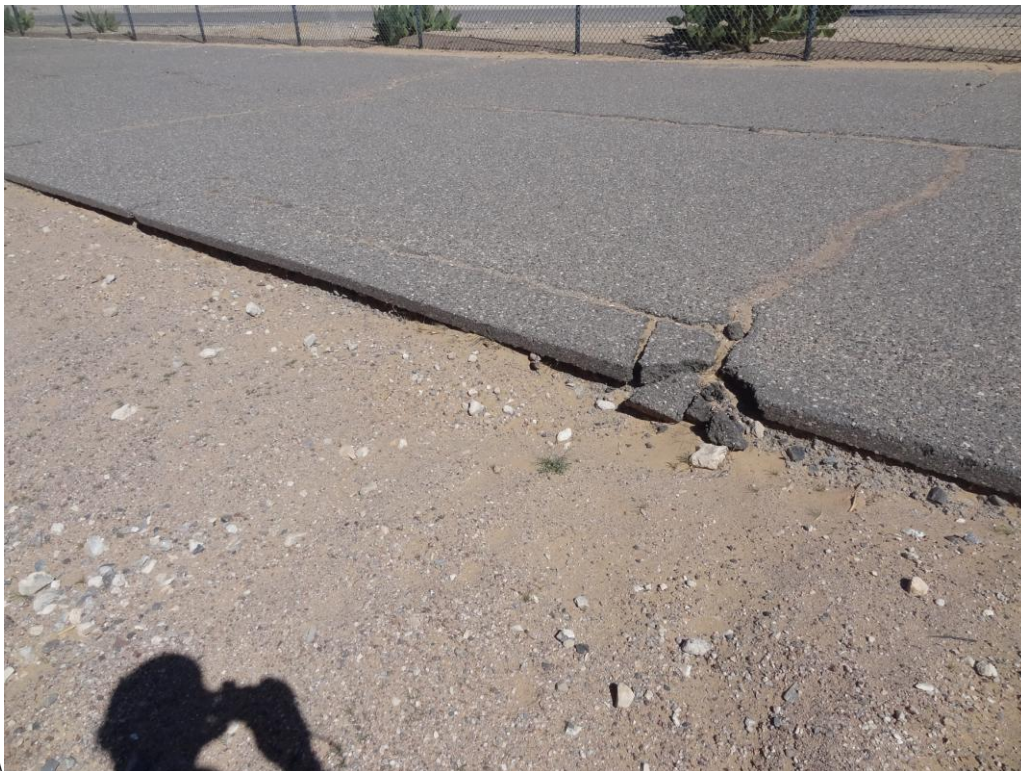
Southern Nevada Correctional Center Site - Site #9994 Description: AC paving in need of replacement.
