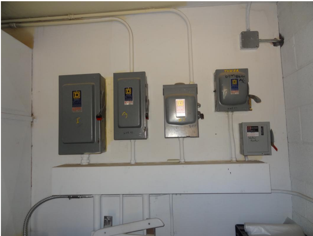
Recreation/ Gym - Building #0186 Description: Electrical equipment in need of replacement.
